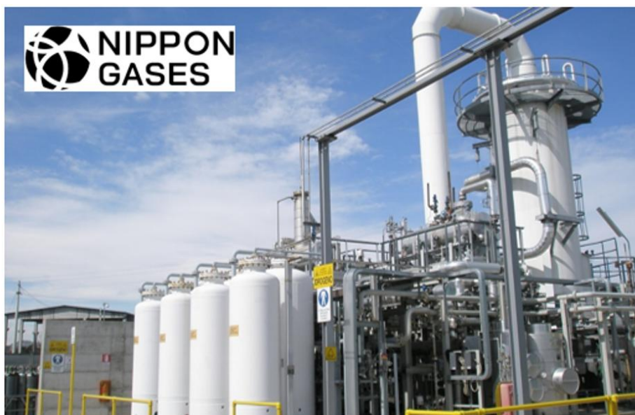
Figure 26. Nippon Gases steam methane reforming plant for the hydrogen production in San Salvo.
