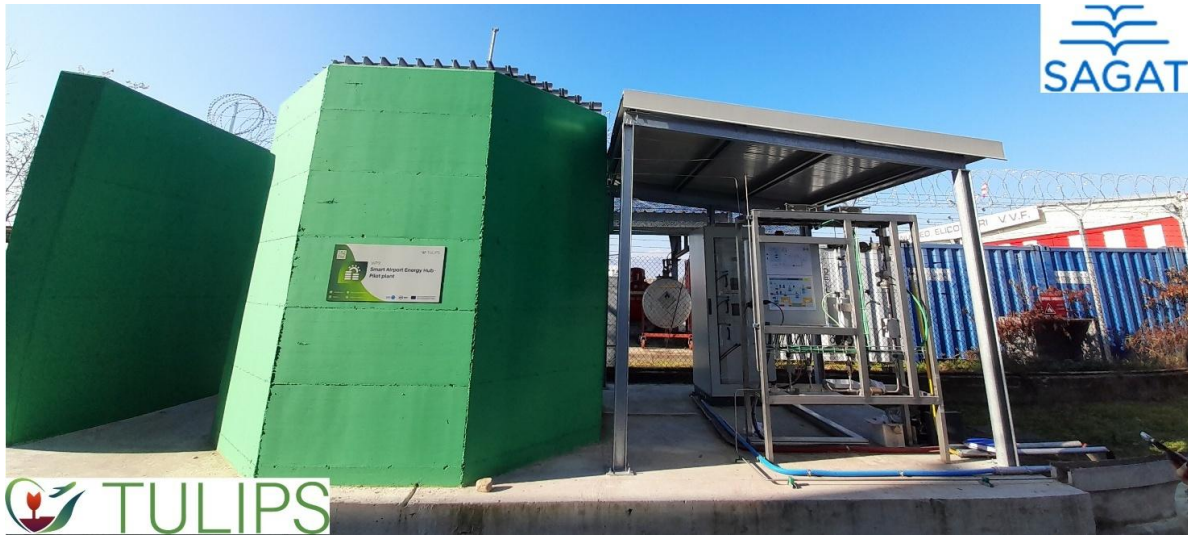
Figure 10: Alkaline electrolyser demonstration plant at the Torino Airport.
